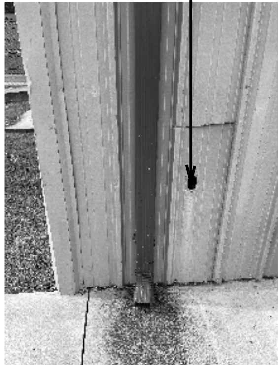
HOLE IN EXTERIOR WALL AT THE SOUTH EAST CORNER OF THE GYMNASIUM BUILDING
