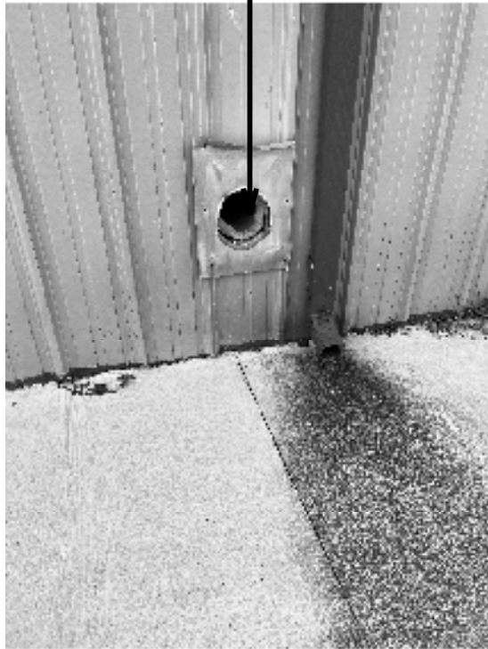
HOLE IN EXTERIOR WALL OUTSIDE OF THE EXISTING LAUNDRY ROOM
