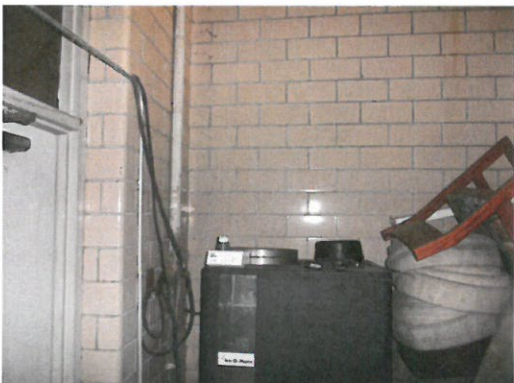
TSI/Pipe/Engine Room (AS-05)
