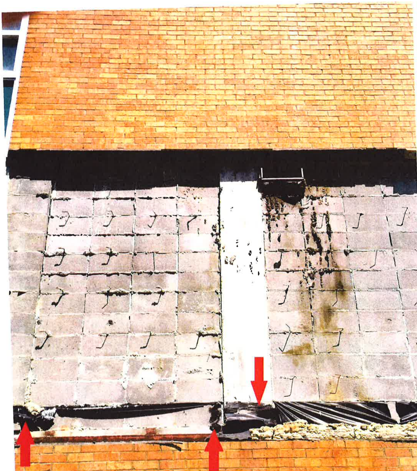
MASTIC ON WALL, COLUMN & VAPOR BARRIER
