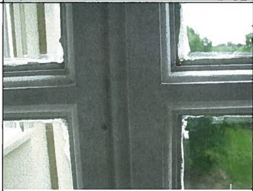
75. Water stain on frame of Unit C3.
