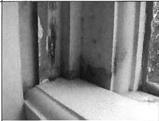
118. Water stain on frame and jamb with mildew on Unit E2.
