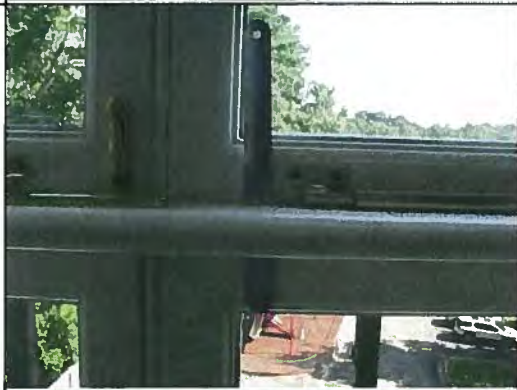
53. Open joint from below casement leaf to interior of lower fixed panel on Unit G.
