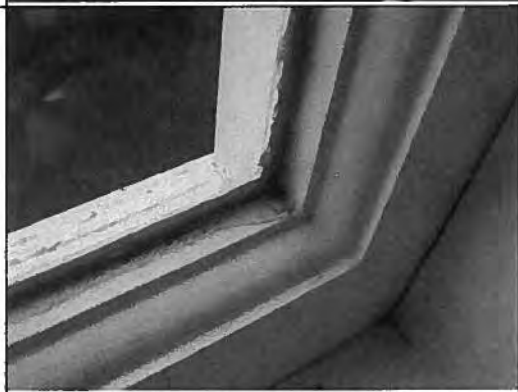
117. Water stain on frame of Unit E2.
