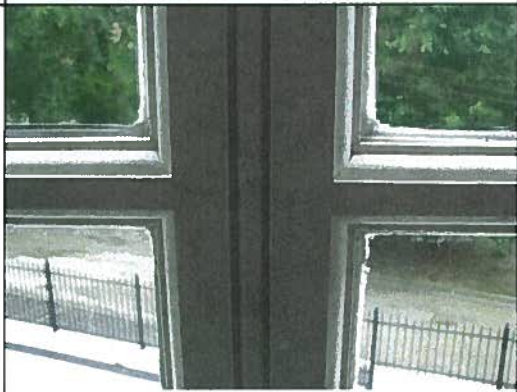
62. Excessive exterior sealant on Unit E3.
