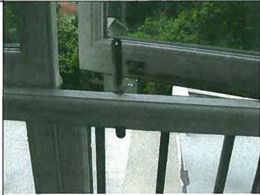
68. Open joint by poor design of Unit H.
