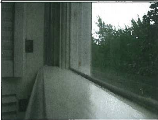
17. Rust at exterior jamb of Unit G3.
