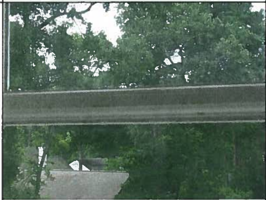
34. Water stain on frame of Unit A2.
