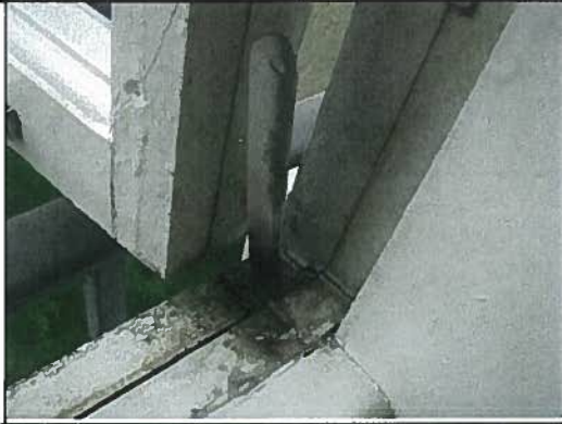
121. Decayed wood in frame of Unit G.
