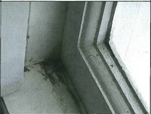
67. Water stain on sill, jamb and frame of Unit B3.
