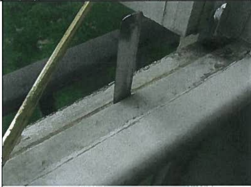
122. Open joint from below the casement leaf to the interior of the lower frame of Unit G.
