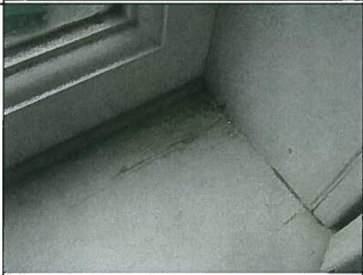
48. Damaged finish of sill of Unit E2.
