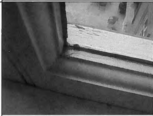
77. Water stain on frame of Unit D3.
